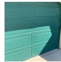
Garage Door Damage
