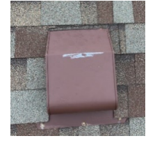
Storm Damage to Soft Metals
